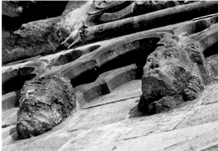
Figure 3: Photo: Archive of the Restoration Workshop of the Nidaros Cathedral (ARW) 1992, taken from [14]. It shows the rapid weathering effects of a part of the Nidaros Cathedral (the frieze from the choir) made of Grytdal soapstone in the 1880s.
